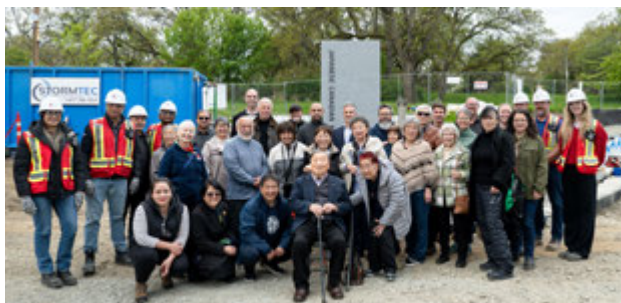
Installation of first granite panel. Members of Victoria Nikkei Cultural Society, Ministry of Attorney General MARB, Ministry of Infrastructure Real Property Division, Chandos Construction.
